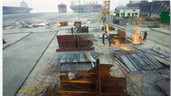
Yard improvements took place mainly in India and Turkey but also in Bangladesh where the PHP Ship Recycling Facility invested heavily into proper infrastructure.
